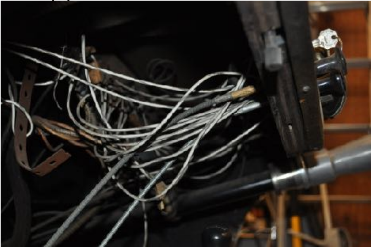
MGTC wiring nightmare
