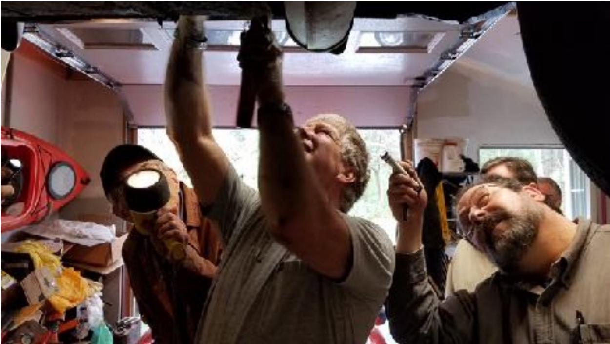
Replacing a fuel tank begins with removing the rear bolts, with Bruce and Ira looking on.
